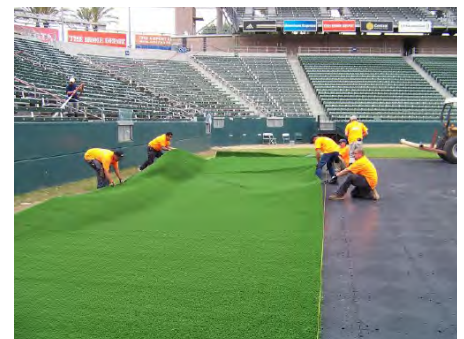
Workers "Pop" the Turf to Allow Air to Flow Under the Turf so it Can Float in to Position
